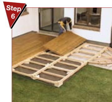
Step 6 Top panels being fixed Slot top deck panels into place and screw to subframe
